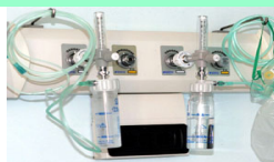
Imp. Gas Medicali UTIC (ASL Catsellaneta - TA, 07)
